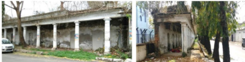
FIGURE 15 CRACKED CEILING AND WILD VEGETATION GROWTH ON THE EXISTING ASTABAL STRUCTURE
