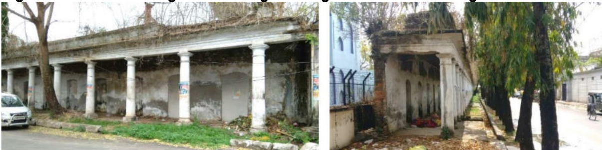
Figure 5: Cracked ceiling and wild vegetation growth on the existing Astabal structure
