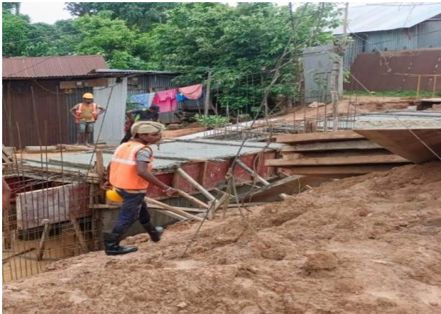
Electrical trench work in progress at Barjala Road. Use of PPEs noted
