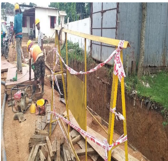
Use of PPEs by workers noted. Shoe needs to be provided to all workers
