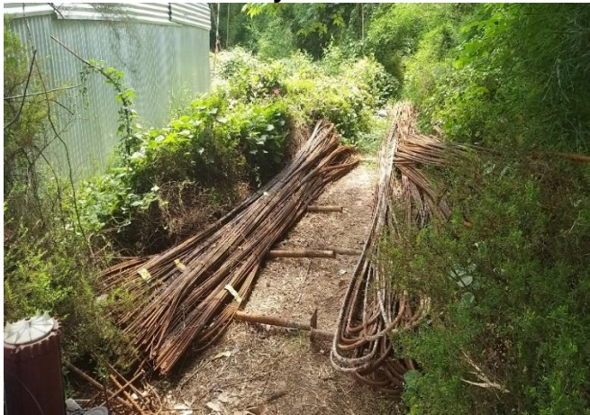
Material needs to be stored above the ground
