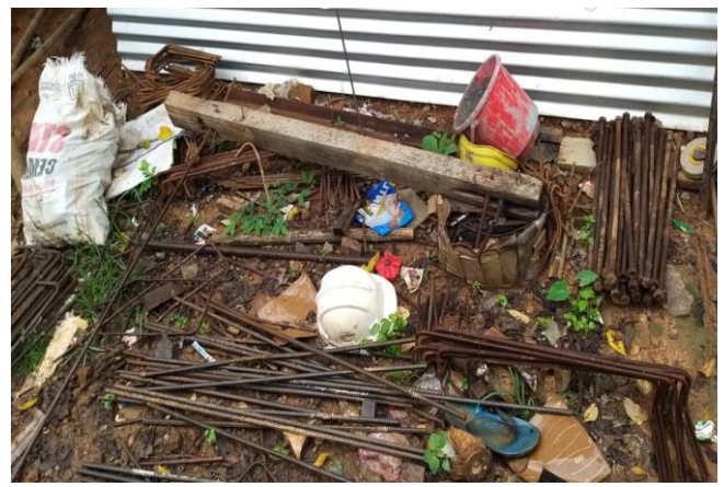
Waste needs to be disposed. Improvement of housekeeping is required
